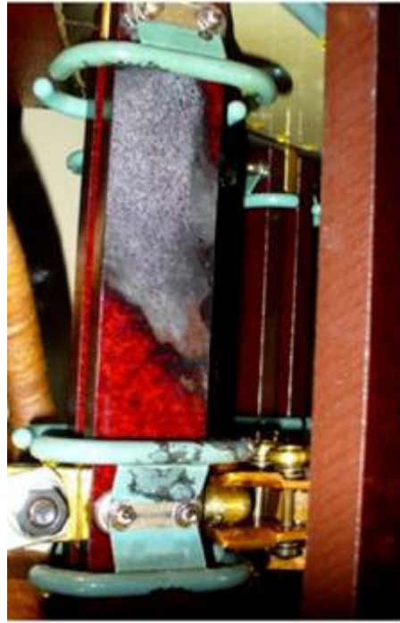
Fig. 4: Example of a power transformer with a fault D1 in oil (on a Bakelite plate), 480 ppm C_2H_2 and no failure observed in service
